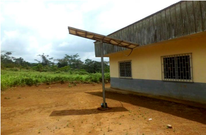
Figure 3: Solar panel at the Big Ngwandi IHC, Mbonge
